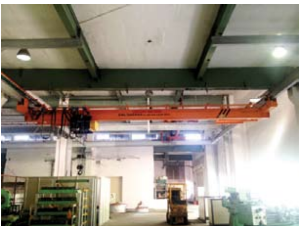
Underslung EOT Crane
