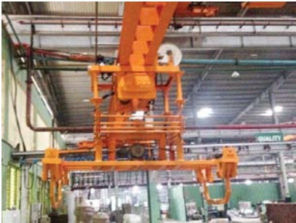
PLC Control Crane with Grabler
